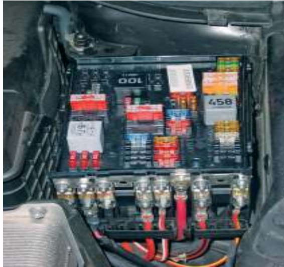
Figure 2-5 Typical fuse box or panel
