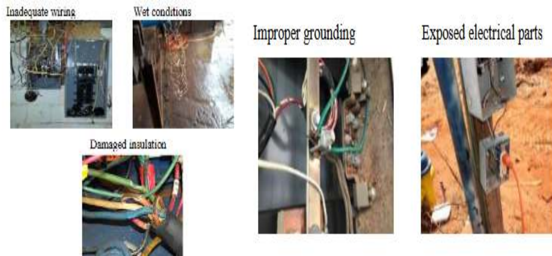
Fig 1.2 Electrical Hazards in Textile Industry
