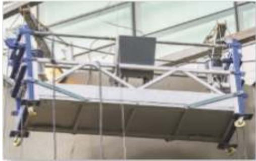
Fig 2.1.2 C) Suspended scaffolds
