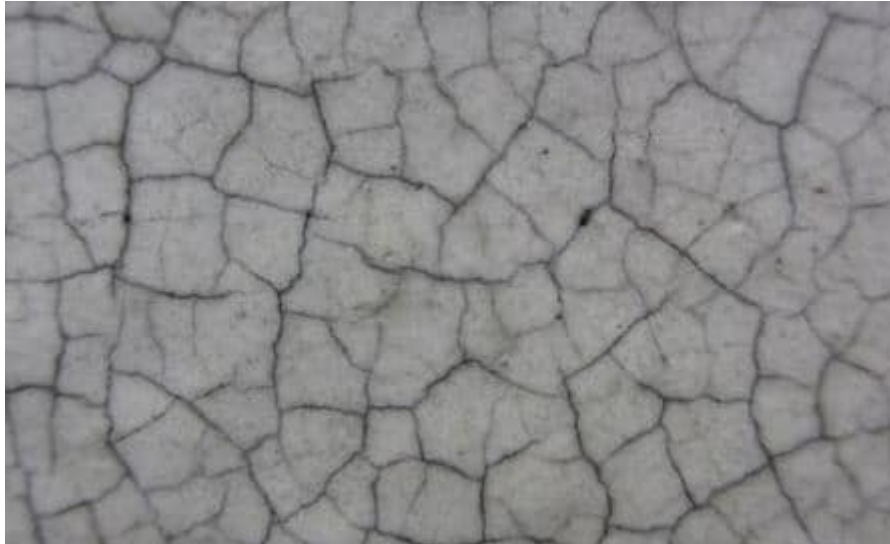
Fig3.2 Crazing or pattern cracking
