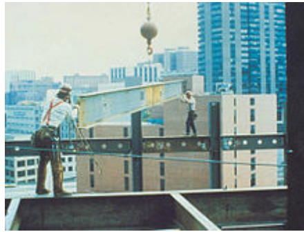
Fig.1.8 At-risk workers without appropriate safety equipment
