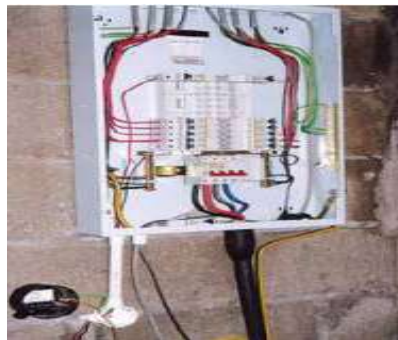
Figure 2.1 Wrong installation of socket out let from distribution board
