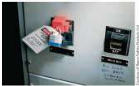
Figure 2.2 Main Switch/MCB Isolation, Lock and Tag
