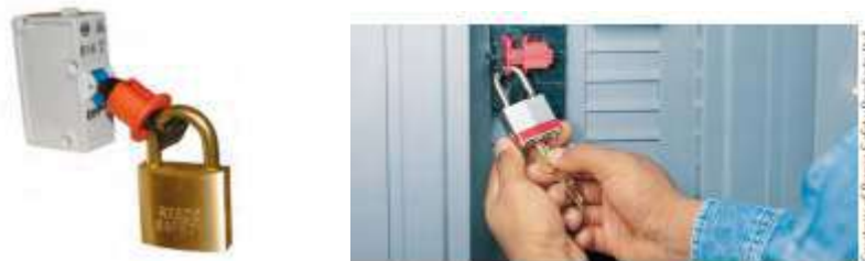
Figure 2.4 Circuit Breaker locking off clip with a padlock
