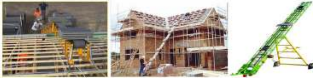
Figure 2.1 Elevator for roof
