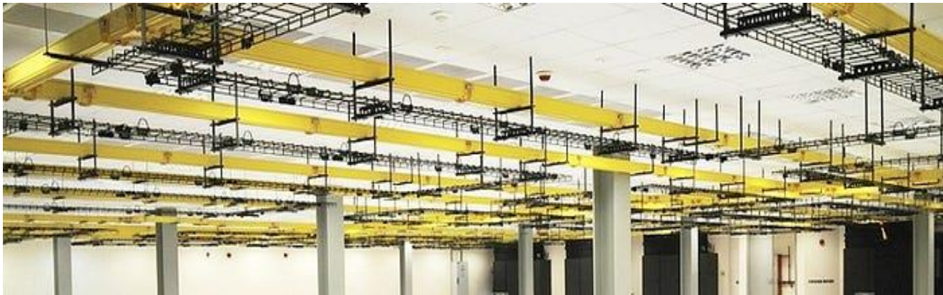
Figure 9 Underfloor Cable Tray
