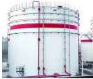
Figure 3.9 Fire water storage tanks
