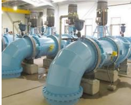
Figure 1.9 Industrial water treatment
