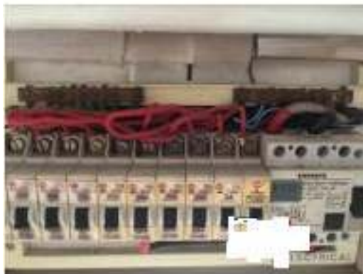
Fig 2. Bad Wiring or loose connections
