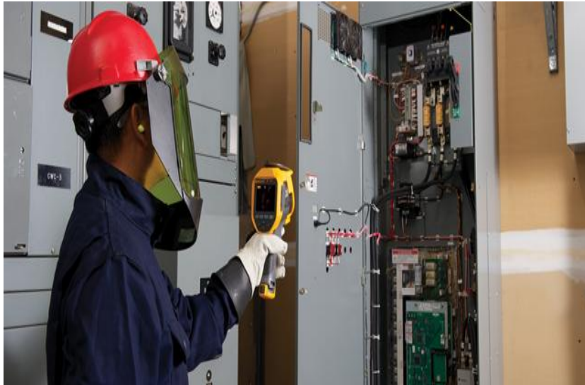
Fig 1.thermography scan of all electrical systems
