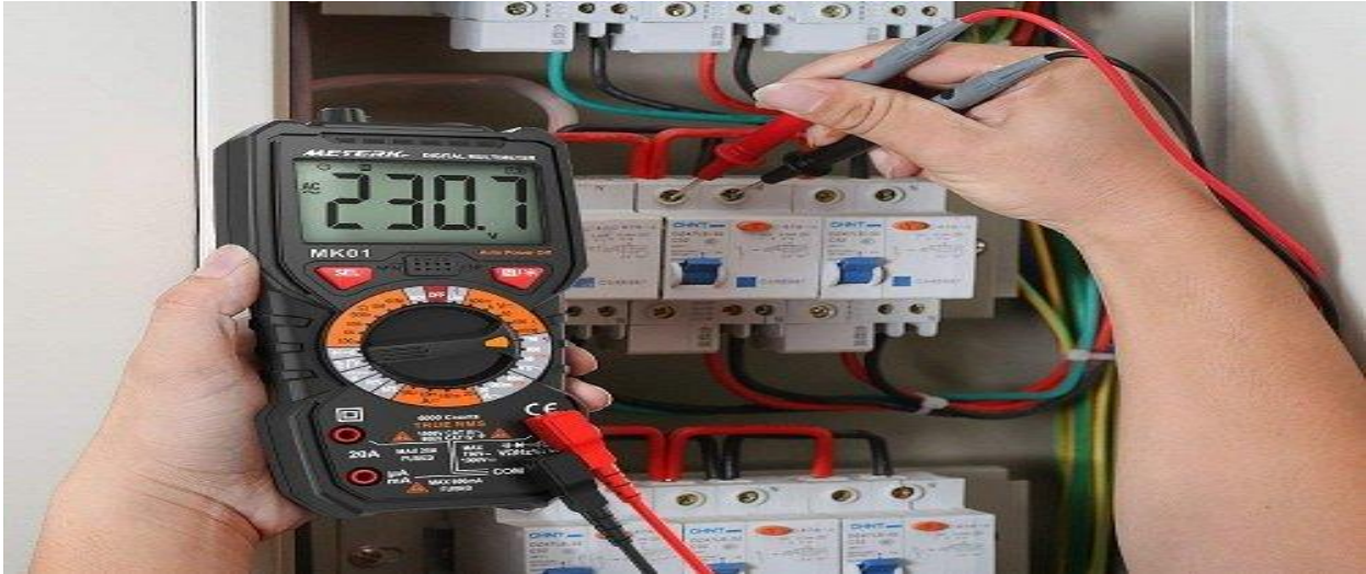
Fig 16. Testing circuit breaker
