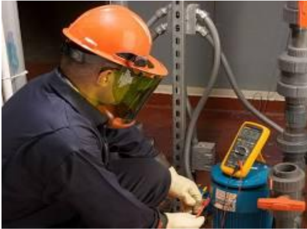
Fig 8. Check single phase motor
