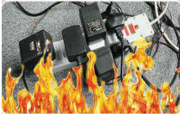
Figure4. 3A danger arises if these extension blocks are overloaded.
